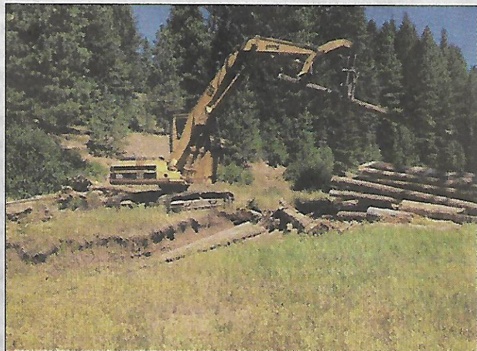
CREWS ARE IN THE Teanaway Community Forest at Indian Creek, creating logjams with woody debris (trees and root wads), part of a restoration project aimed to deliver several benefits. Here the excavator is at work creating logjams for the creek.
